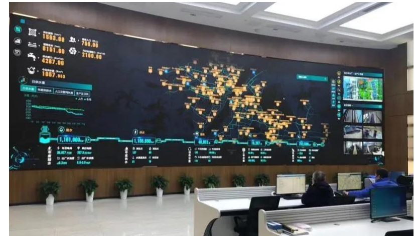
Fig 8. Intelligent water system from Wuhan Water Group Limited Company
