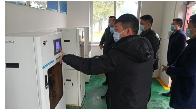
Fig 9. The operation of sewage treatment facilities were inspected in Huangping county, Guizhou province
