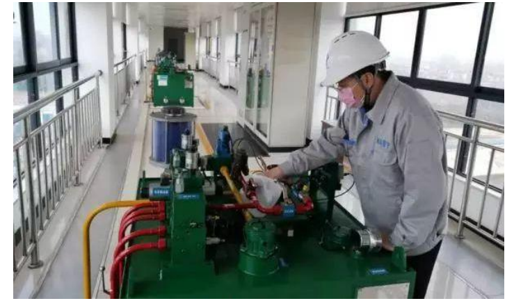
Fig 6. Patrol gate station of the South-to-North Water Diversion Project in YuZhou, Hubei province
